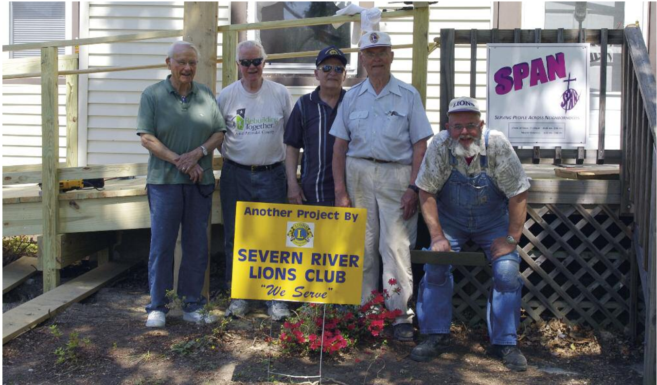
Lions Ken Tschantre, Rhine Jager, Bill Stack, Dale Strait and George Council take a break from building the SPAN handicap ramp.
